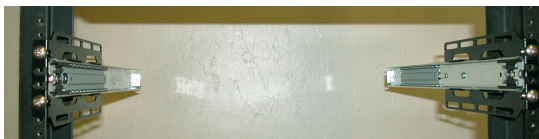
Side rails mounted in a 19" rack.
